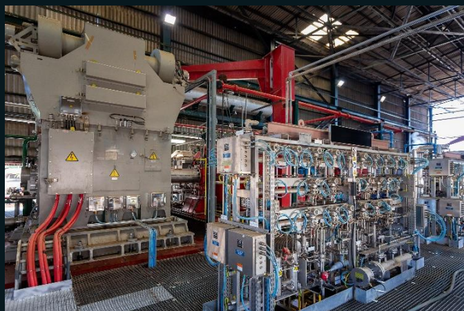
Repsol's Puertollano Olefins Plant in Spain
