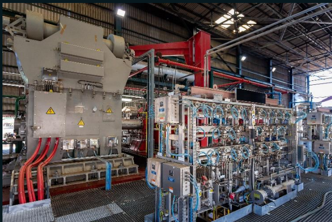
Repsol's Puertollano Olefins Plant in Spain
